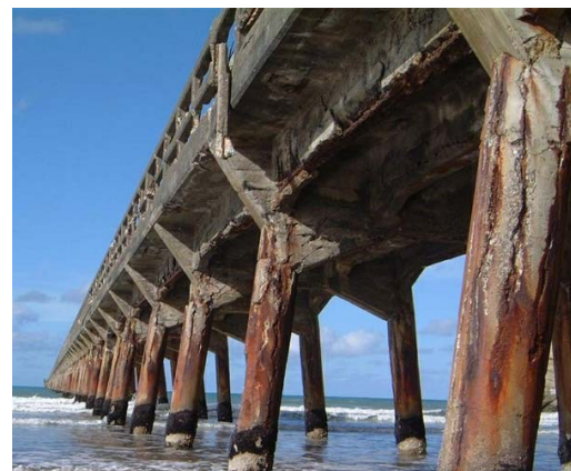
Figure 5.10. Example marine reinforced concrete structure suffering from corrosion ( www.goldseal.co.nz/marine2 )
