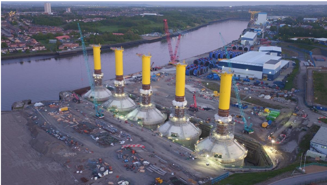
Figure 21. Construction of concrete gravity foundations for offshore wind in a dry dock at Blyth
