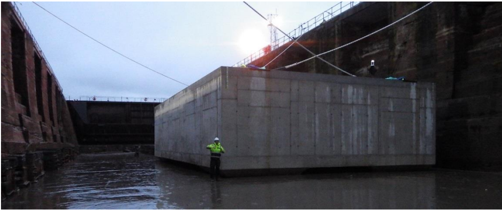
Figure 53. A complete concrete gravity substructure built in a dry dock, awaiting float-out
