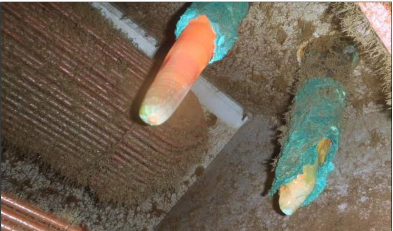
Figure 16: P2 heat exchanger and their associated anti-fouling copper anodes (marine growth is on the edge of acceptable level and duty-cycle of anti-fouling system was subsequently increased to improve anti-fouling characteristics)
