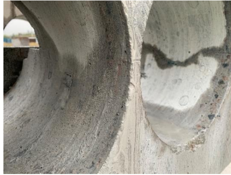
Cores extracted across the precast connection
