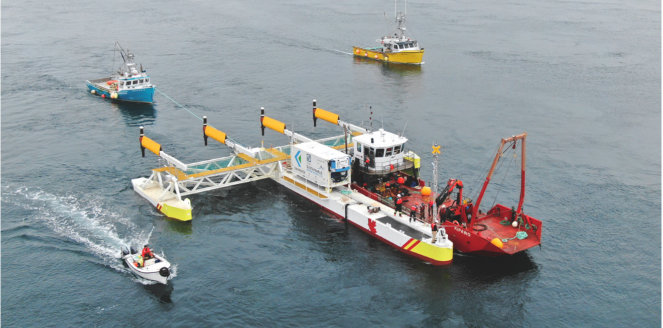
SMEC Plat-I Installation, Grand Passage, Nova Scotia, Canada Courtesy: Sustainable Marine Energy (Canada) Ltd. (SMEC)
