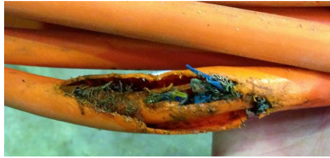
Figure 4 – Example of failed cable
