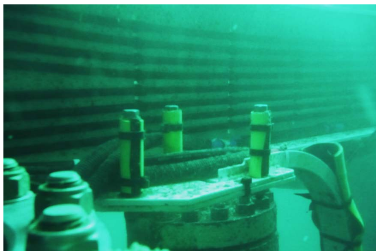
Figure 8 - Cables and hydraulic hoses on robust, open and accessible cable trays
