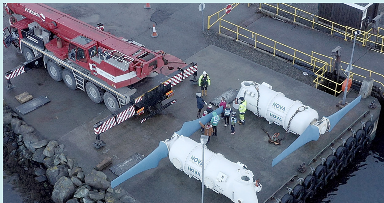
EnFAIT turbines 5 and 6 inspected by pupils from Cullivoe Primary School before installation (Credit: Nova Innovation)
