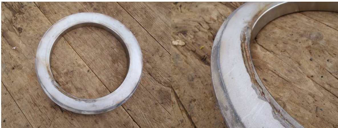
Figure 7 – Crevice corrosion on a 316ss Spacer piece due to internal seawater in pipeline system.
